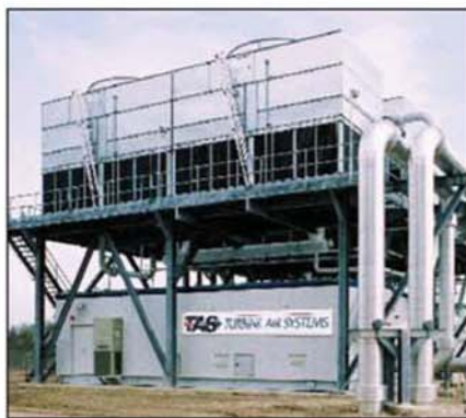
An inlet chilling plant in Brazos valley, Texas
